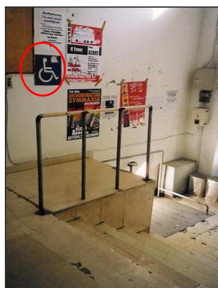
Fig. 14-6: A simple lift mechanism at the Medical University of Athens, but the railing is missing!
